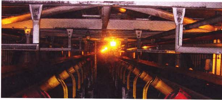
L-beams and conveyors belts are areas where dust collection can result in potential hazards.
